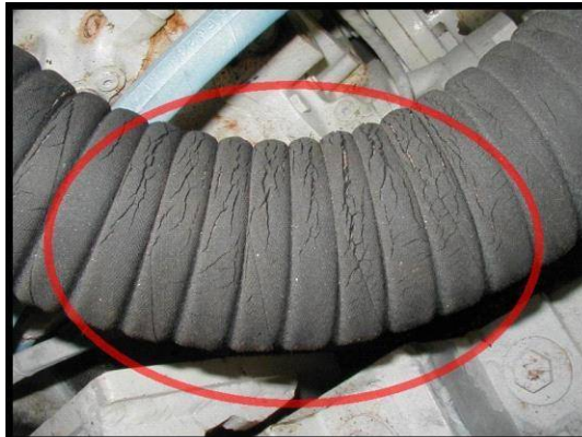
Cracked raw water hose
